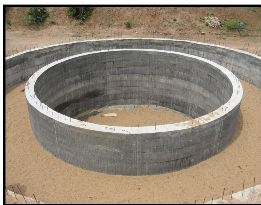
Recharge Shaft in namakkal District in Tamilnadu
