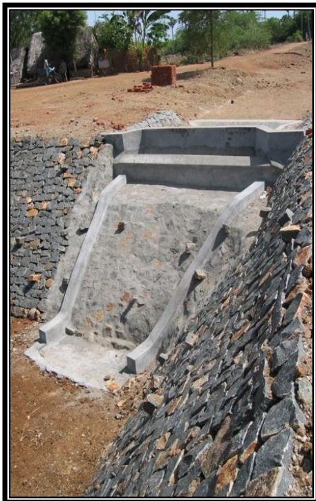
8.19 (a) Settling Basin
